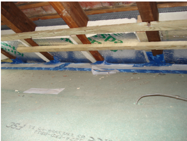
High performance PUR fitted between rafter to provide a continuous insulated envelope over the top of the external walls.
