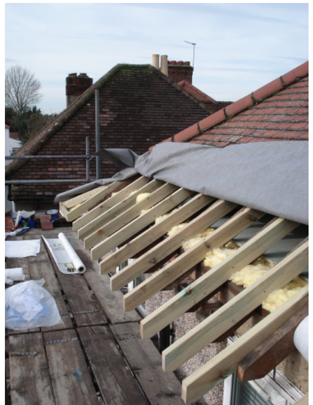
High performance PUR fitted between rafter to provide a continuous insulated envelope over the top of the external walls.
