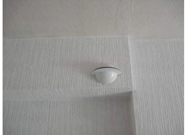
Supply air diffuser from HRVU
