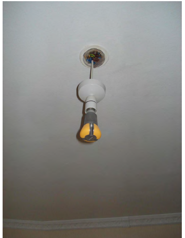
Low energy light bulbs throughout
