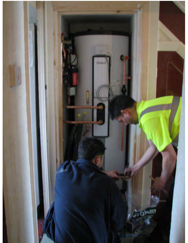
Solar thermal cylinder installed in under-stair cupboard
