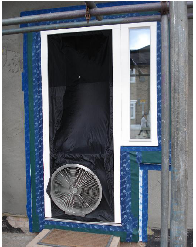
Door fan to front door during airtest . Airtightness tapes and membranes continuous are from door and windows to parge coat.
