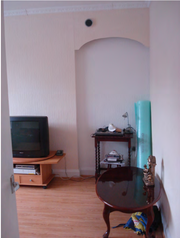
Internal wood fibre insulation to party wall either side of chimney breast
