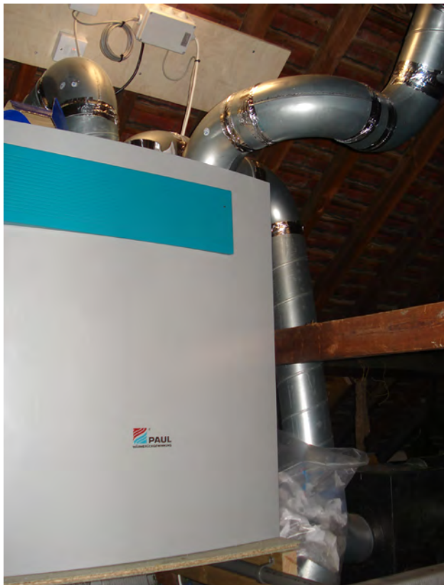
Paul Novus 300 heat recovery ventilation unit (HRVU )to attic
