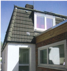
ECD's retrofit of a semi in Crawley included overcladding the pre-cast concrete walls on the ground floor, internally lining the mansard to retain the roof tiles and introducing Passivhaus-standard windows.
